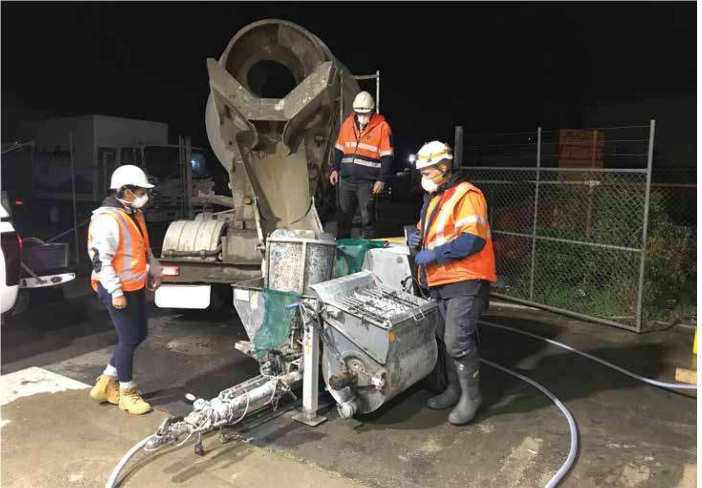
Interflow's team worked through the night to complete the critical wastewater project.
