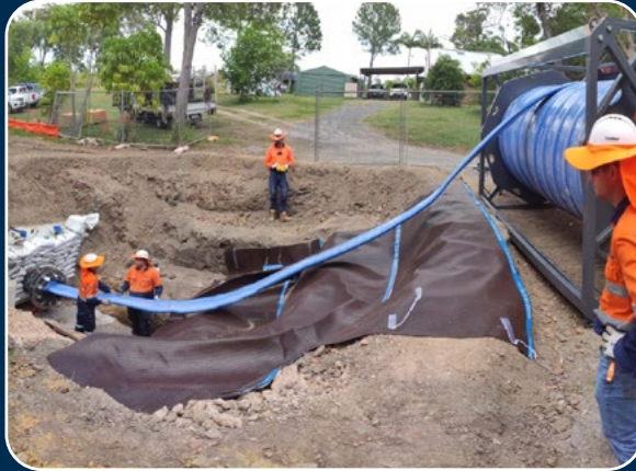
Primus Line is winched through the pipe section from a compact, pre-wound spool.
