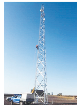
Balonne Shire will utilise existing grain silos and water towers plus 45 new towers to deliver fast internet out west.
