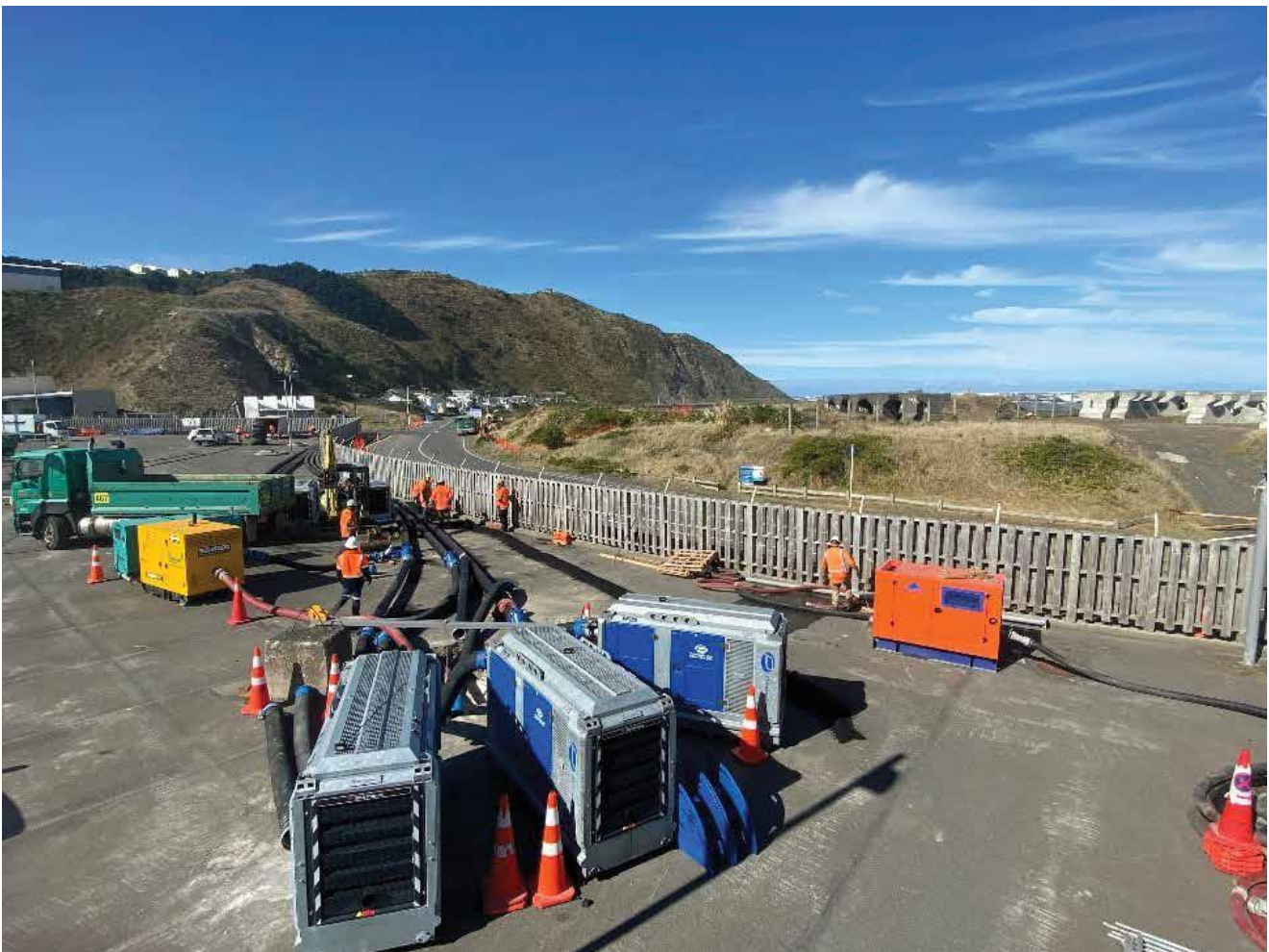
Pumps and temporary piping were used to by-pass the corroded section of pipe.
