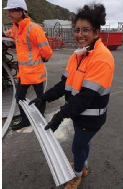
A durable, long-term solution: Saadia Ali with a section of the PVC used to line the interceptor.
