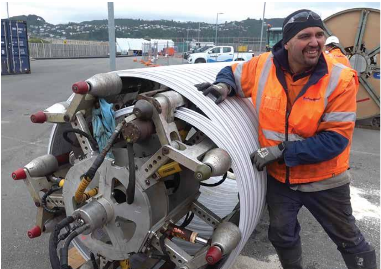
An above-ground demonstration of the pipe lining machine by Adam, a foreman for our contractor, Interflow, showed how the plastic compound spirals forward and is glued into place as it advances through the host pipe.
