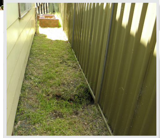
Depression visible midway along the trench
