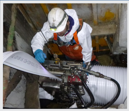
Installation of an SPR™ EX - Expanda Pipe liner in a deteriorated stormwater pipeline
