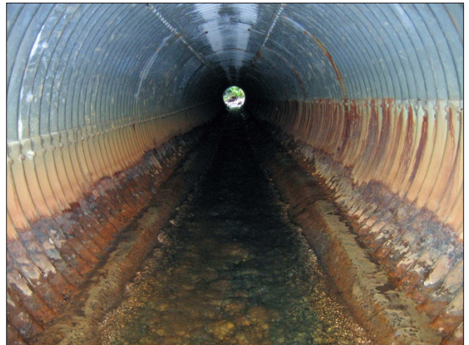
Figure 5: Concreting the invert of a culvert can extend its life, but ultimately moves corrosion and abrasion problems further up the wall.
