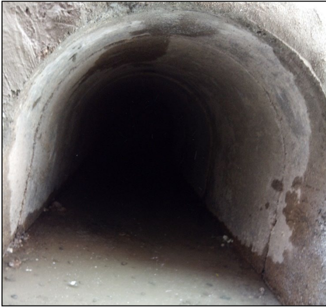
Figure 10: Non-circular culvert subject to deterioration and heavy siltation
