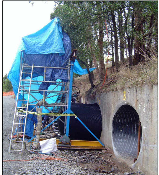
Figure 9: Installing a Ribline liner in an 1830mm diameter culvert. Note the culvert in the foreground has been completed, including grouting and epoxy end sealing.
