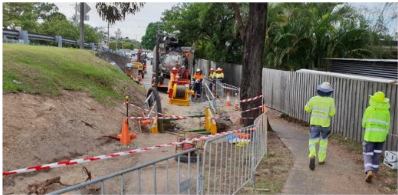
Figure 10. Southern end of the Eastern Force Main – the need to maintain pedestrian access around the site was critical
