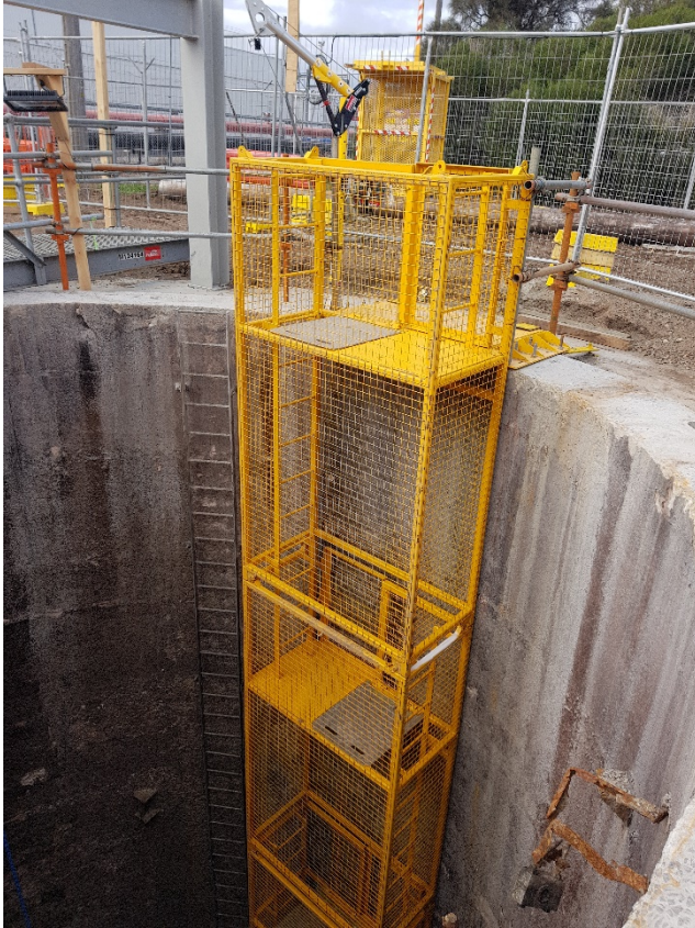
Figure 3: Caged safety ladder in situ in manhole.
