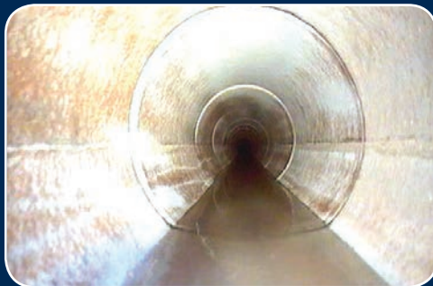
After cleaning, the pipe walls are clear and smooth and the hydraulic capacity of the pipe is restored.
