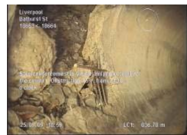
Poor condition. Action needed to prevent ground subsidence and possible collapse.
