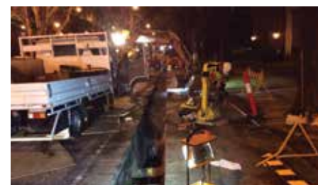
The St Kilda Road Main Renewal Project involved the replacement of 1.4 km of cast iron main.
