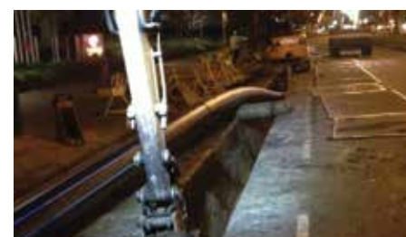
Work was carried out at night, replacing 200 m sections at a time.
