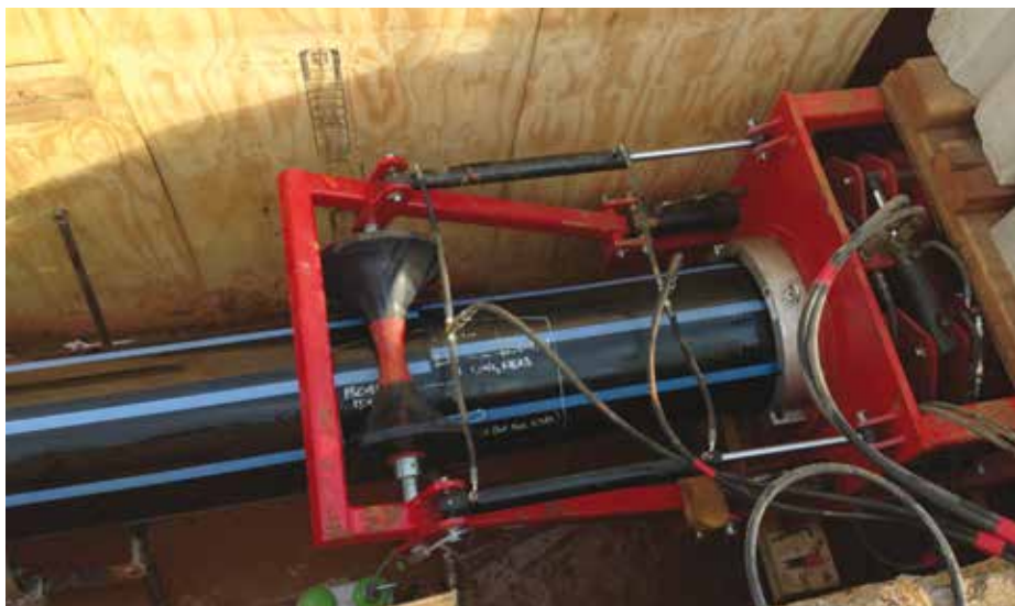
New PE pipe being inserted into the host pipe to be rehabilitated.
