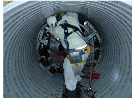
Rotaloc restored the structural capacity of the original pipe making it safe to enter the relined sections of pipe.
