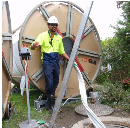
The PVC profile was delivered to site on spools and fed into the Rotaloc winding machine in the sewer below.
