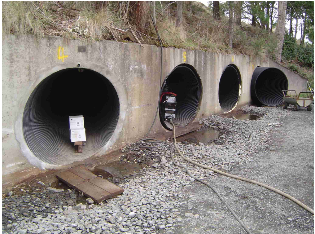
Culverts with liners in various stages of completion. The culvert on the left has been grouted and end sealed and is virtually complete. The centre two culverts have yet to be grouted, while the far culvert has yet to be trimmed.
