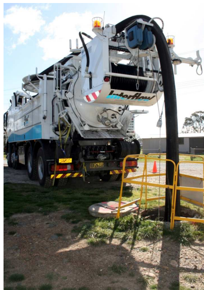
Interflow's Super 2000 Recycler Cleaning truck in operation in Chatsbury St, Goulburn, NSW.
