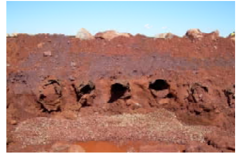
Deteriorated culverts prior to renewal with Expanda.
