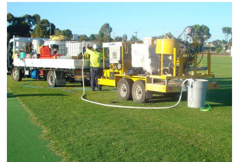
The small footprint of the Interchem™ CAC unit allows the work to be undertaken with minimal disruption to the community
