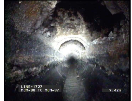
Pre lining CCTV shot inside the MCM sewer; the pipe is in poor condition and sections of the original pipe wall are missing.
