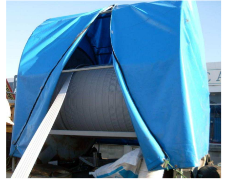
A thermal cover and frame were fabricated and placed over the spool of profile to maintain the temperature of the PVC liner above 15°C
