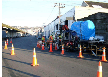
The small footprint of the Expanda installation site meant that work could be performed from access chambers located on roads whilst the road remained open to traffic
