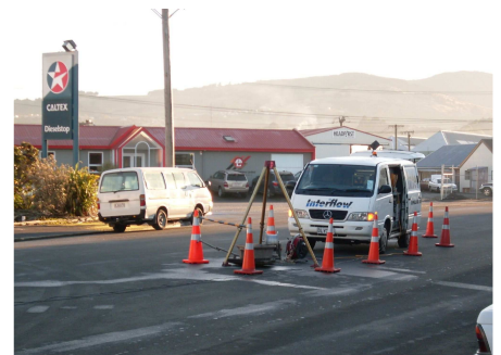
A CCTV crew performs a final survey of the pipeline after the pipe has been lined.
